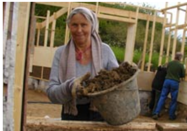
Mariann Wickander lives in Ekoby Baskemölla. In the picture she is building walls with wood-chip clay for the day care in the village.
